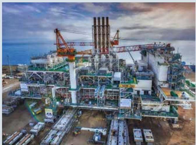
Offshore Crane, Shah Deniz Phase 2, Azerbaijan
