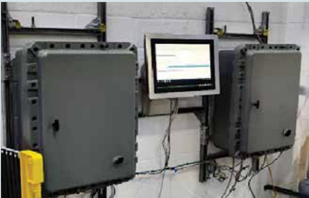
Process Deck Mercury in Gas and Condensate Analyzer Systems for Pegaga Development Project
